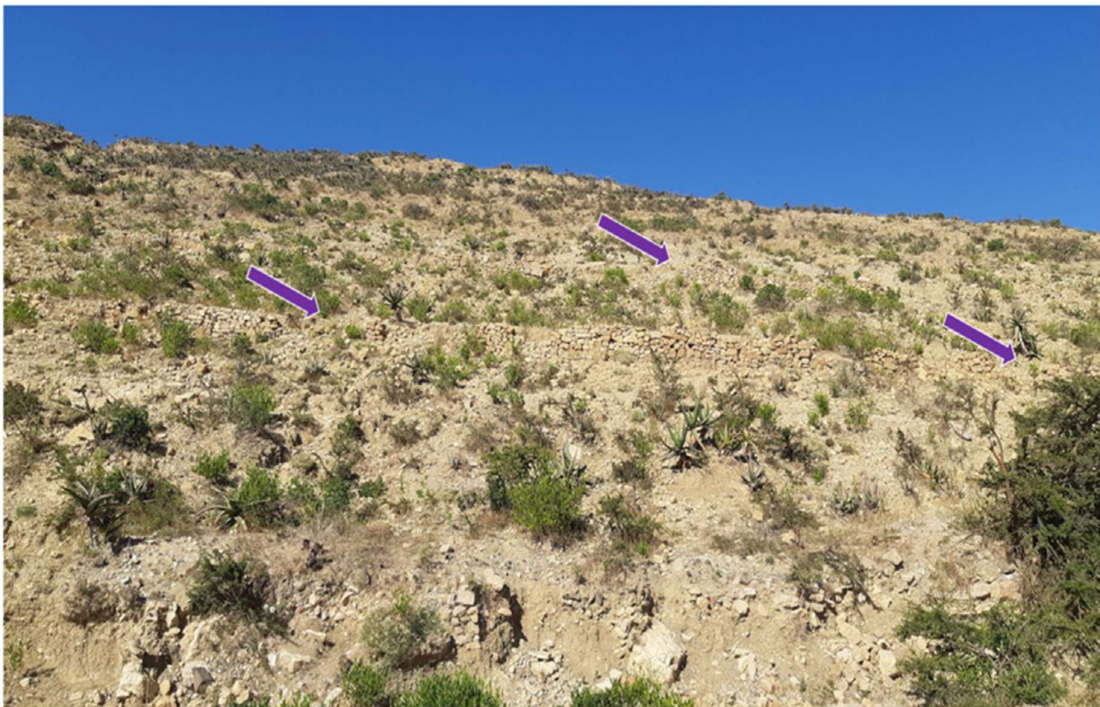
Figure 6. Partial view of the collapsed physical SWC structure at Ala Asa Village. The arrows indicate the fallen stones due to the war.
